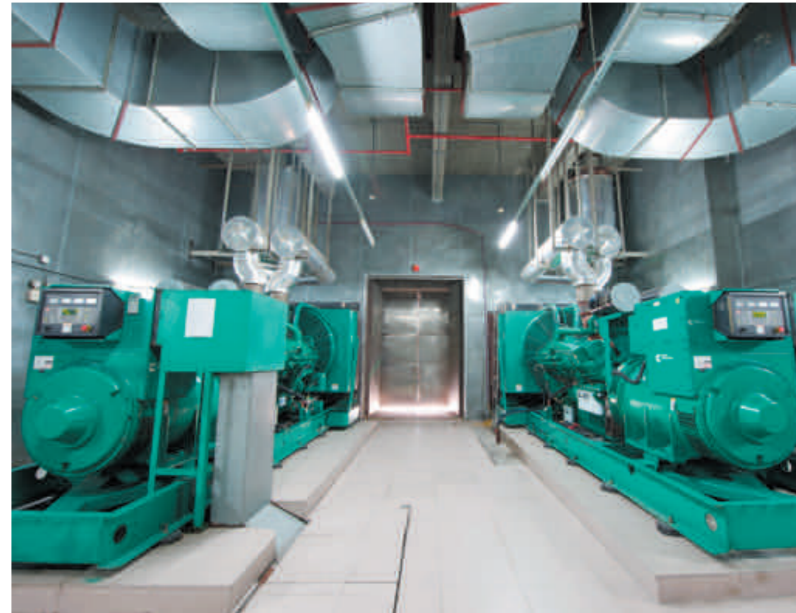
Generators in our plants.
