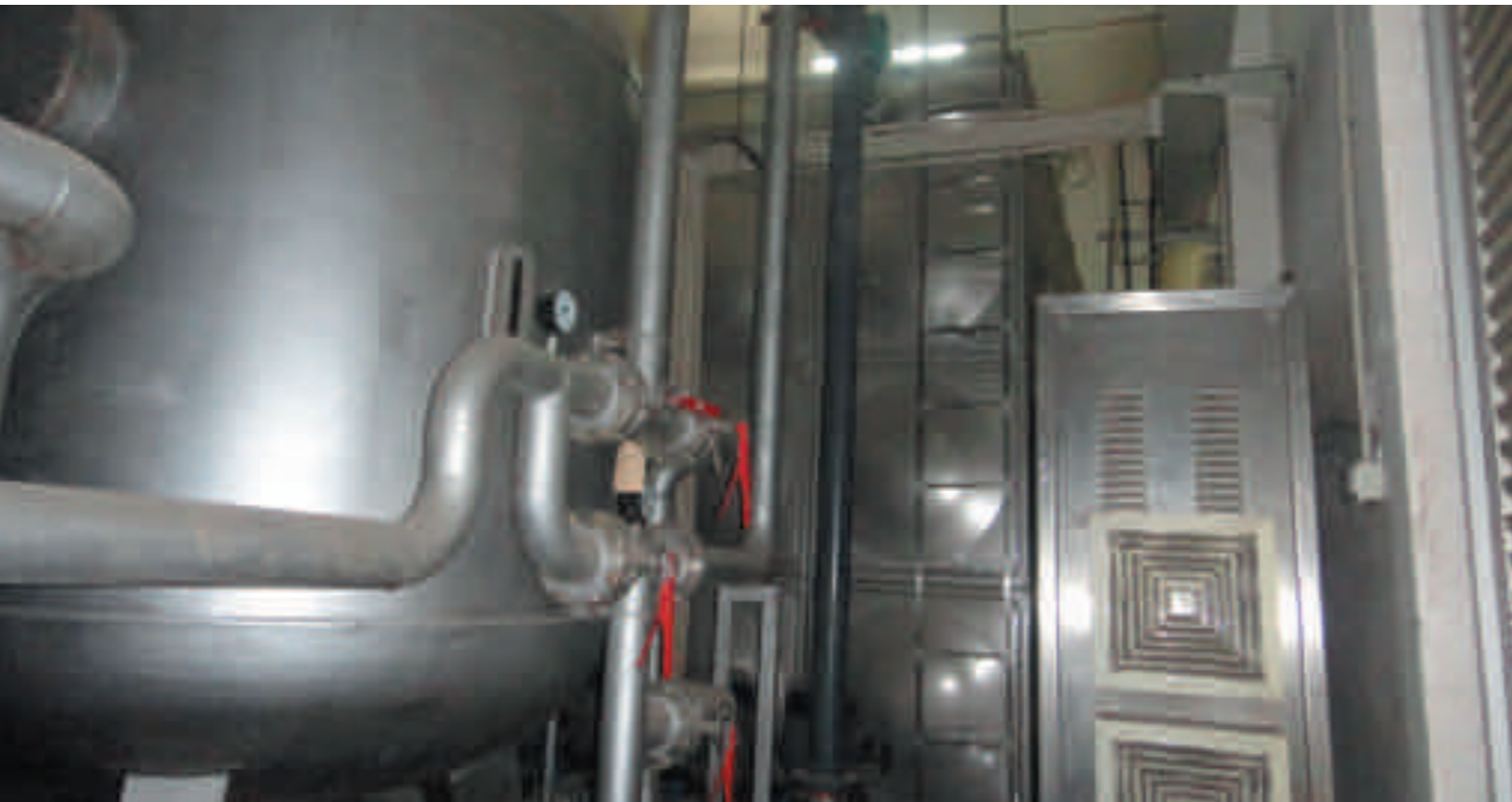
Recycling system for landscape irrigation and toilet flushing.
